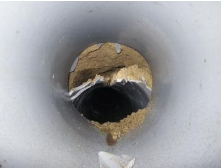
PVC pipe collapsed
