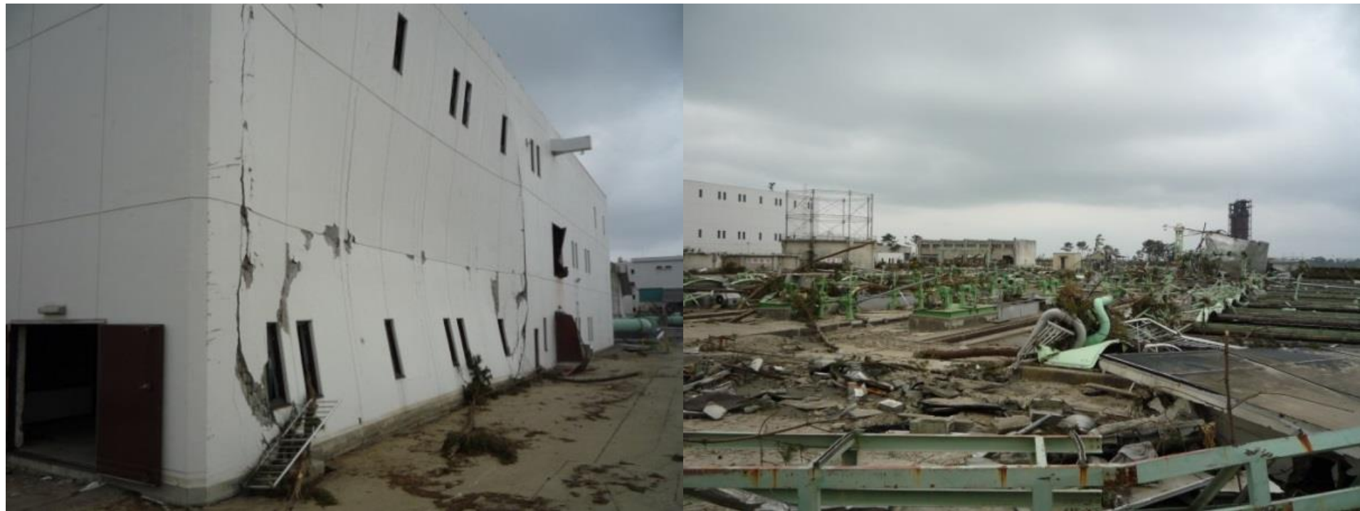
PS building's wall, yielded
