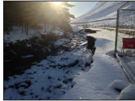
Major Erosion of A591, a major Lake District transport route
