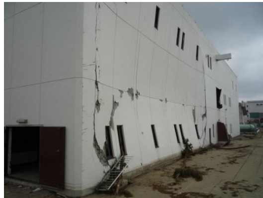
Picture 4.2: The pumping building's wall bent by the tsunami.
