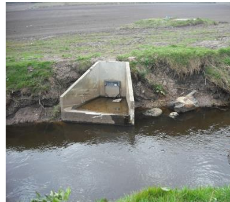
Figure 1: Example of poorly situated outfall with bank protection washed out and eroded because river previously meandered across this field before being straightened and recent high flow events instigated channel change towards a historical planform
