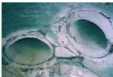
Picture 1: Damage Occurred between the Sewer Pipes
