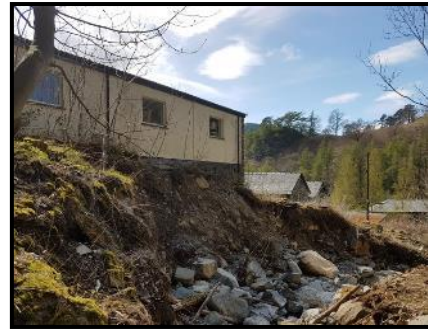
Significant erosion adjacent to UU’s Catchment and Woodland office
