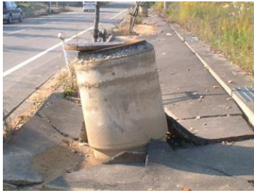
Picture 2: Manhole Floating because of Liquefaction Phenomena
