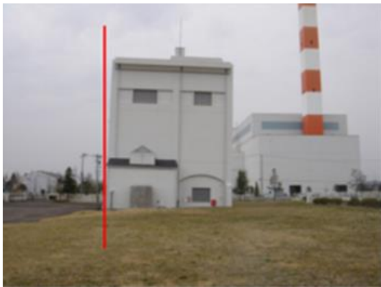
Picture 3.2: The damage of pipeline facilities and inclined pumping building
