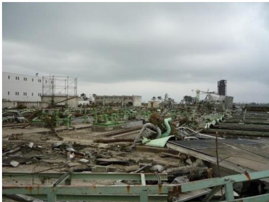
Picture 4.1: The damaged primary sedimentation tank.
