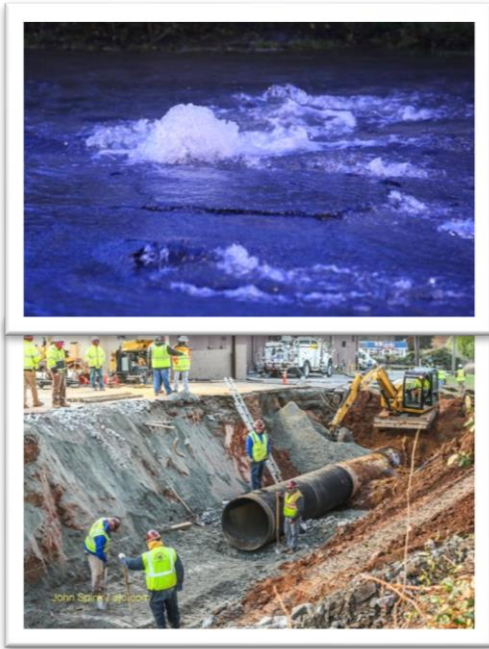
Figure 6. Water main break and repair
