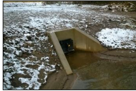
The final result – an outfall located in a less active section of channel, designed by contractor to be set back from main channel and have natural banks as far as possible.
