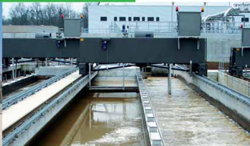
Traveling bridge with grease and grit scraper
