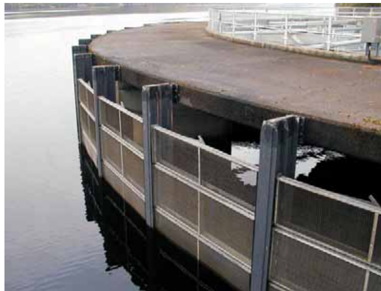
Figure 6: Mesh intake screen at Foyers Pumped Storage Facility / Loch Ness (Scotland) (photo: Scottish and Southern Energy)
